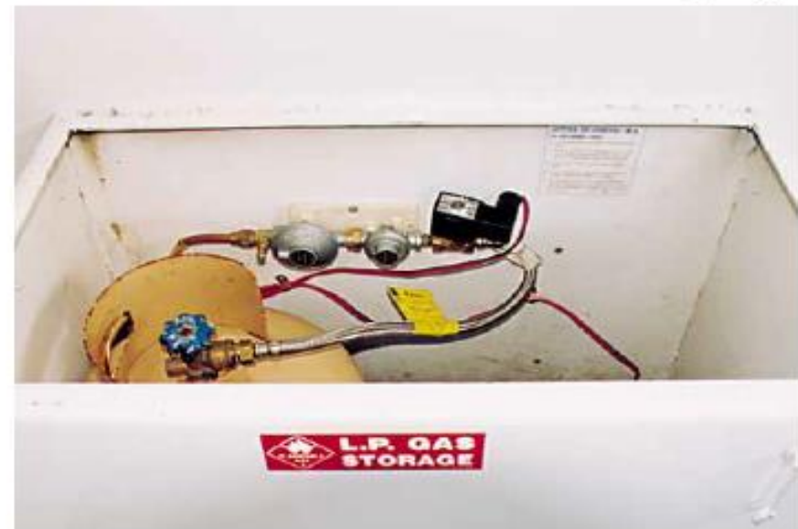
LP gas storage
